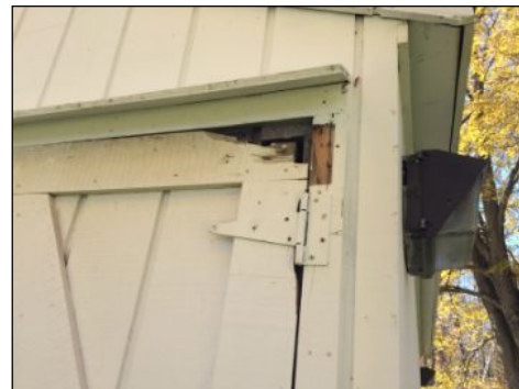
Exterior doors have rot and deterioration which need repair or replacement.
