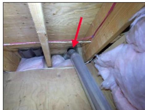
A section of ducting is separated in the attic and needs repair.
