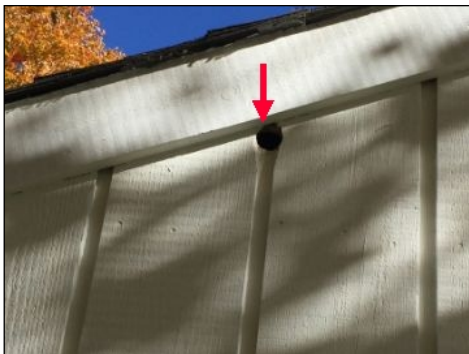
There are holes from wood peckers which need repair.
