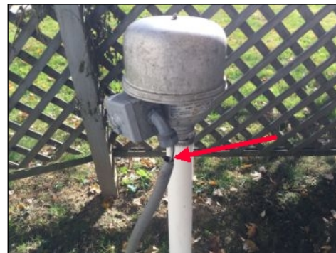
Electrical conduit serving lighting is separated which needs repair.
