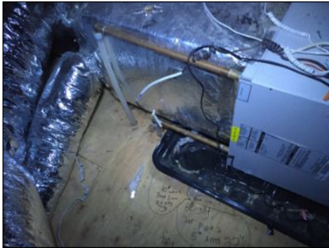
Recommend insulating hydro air heating supply and return lines in the attic.
