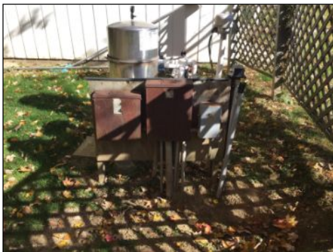
Sub panels and timer serving pool equipment are rusted and deteriorated which need review, repair, and or replacement to ensure integrity.
