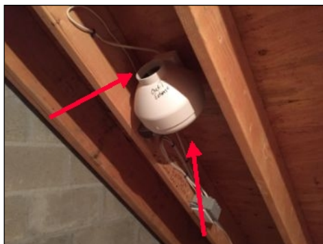
Master bathroom exhaust fan lacks ducting which needs completion to ventilate bathroom.
