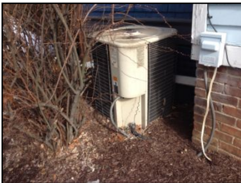
Grading is over base of condenser which needs clearance created to prevent condition conducive to deterioration.
