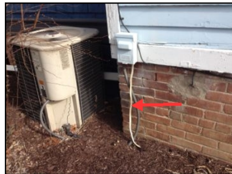
Electrical serving condenser is exposed and needs water proof conduit and connectors.
